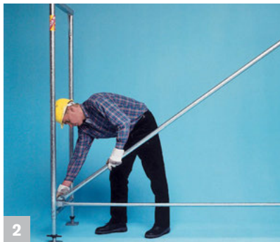
2 Safe and inevitably plumb-vertical erection already after assembly of the first bay
